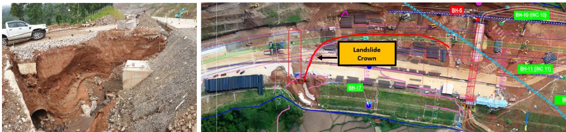
Figure 1. Landslide in STA 21+200 Cisumdawu Toll Road
