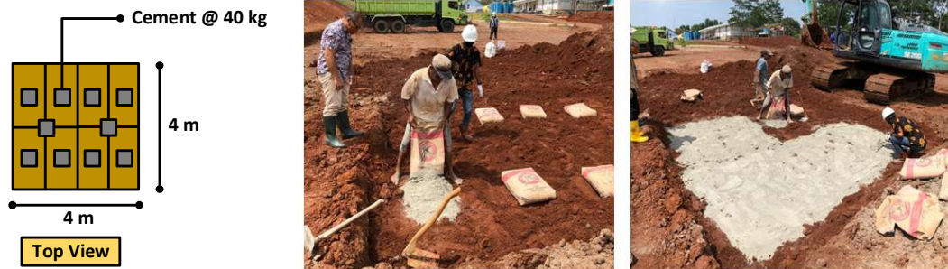
Figure 24. Cement is placed for every 25 cm of soil thickness inside the trial mockup area
