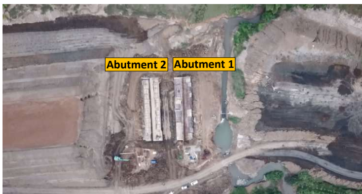
Figure 9. Aerial view of the bridge development area after the lower structure has been fully completed
