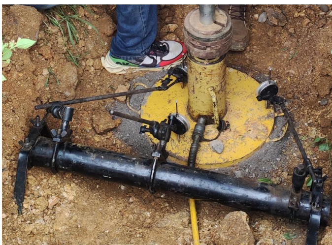
Figure 4. Reference beam used for plate load test is too near the bearing plate.
