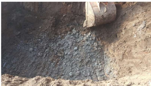
Figure 6. Geoframe's subgrade condition
