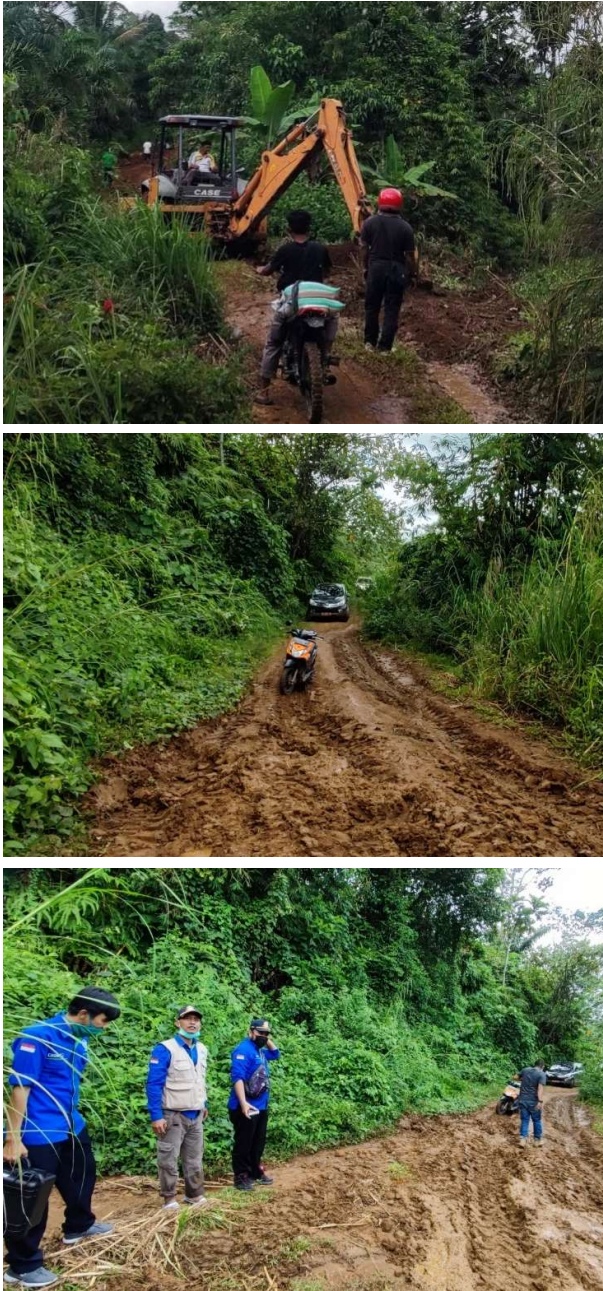
Figure 6. Location of landslides at MAN 4 Timboabu, West Pasaman, West Sumatra
