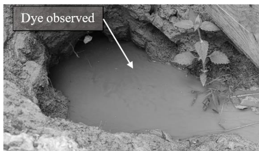
Figure 17. Observations on the soil pipe during the dye test
